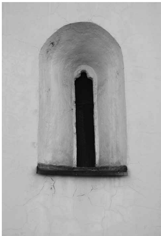
5. Kloštar Ivanić, crkva sv. Marije, zvonik, prizemlje, sjeverni zid, prozorski otvor (foto: M. Cepetić Rogić) / Kloštar Ivanić, church of St Mary, belfry, ground floor, northern wall, window opening (photo: M. Cepetić Rogić)
