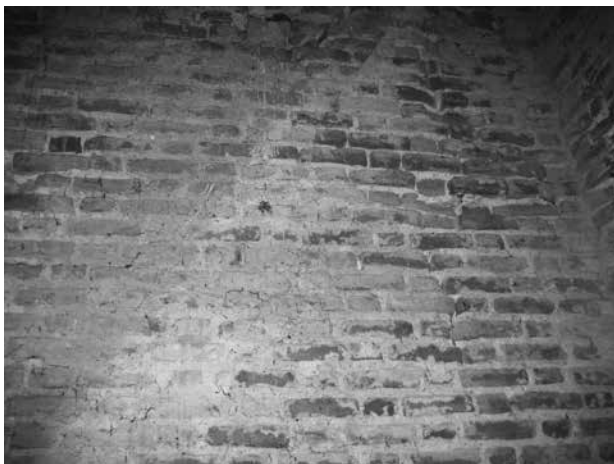
7. Kloštar Ivanić, crkva sv. Marije, zvonik, treći kat, sjeveroistočni kut, razlike u zidu (foto: M. Cepetić Rogić) / Kloštar Ivanić, church of St Mary, belfry, third floor, northeast corner, differences in brickwork (photo: M. Cepetić Rogić)
