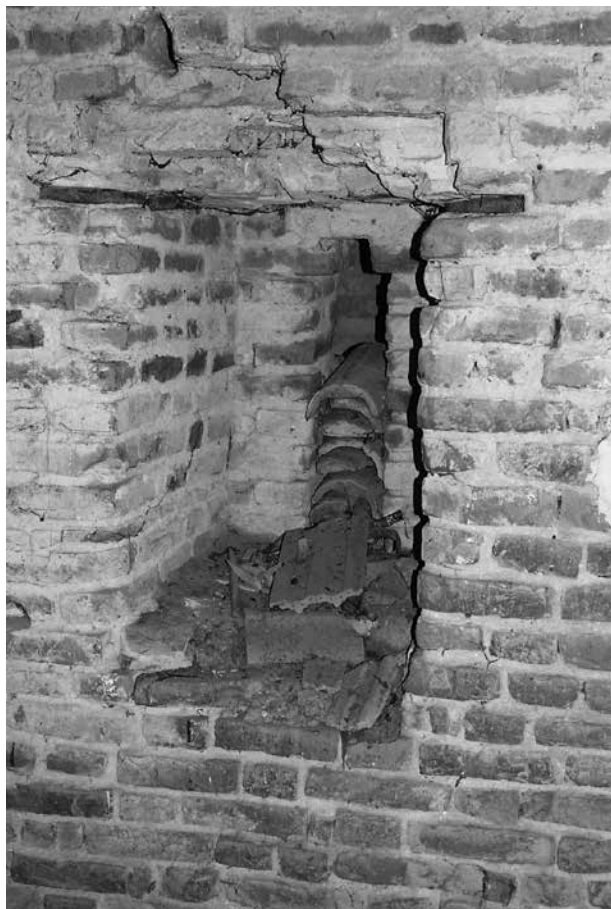
6. Kloštar Ivanić, crkva sv. Marije, zvonik, prvi kat, istočni zid, prozorski otvor (foto: M. Cepetić Rogić) / Kloštar Ivanić, church of St Mary, belfry, first floor, eastern wall, window opening (photo: M. Cepetić Rogić)
