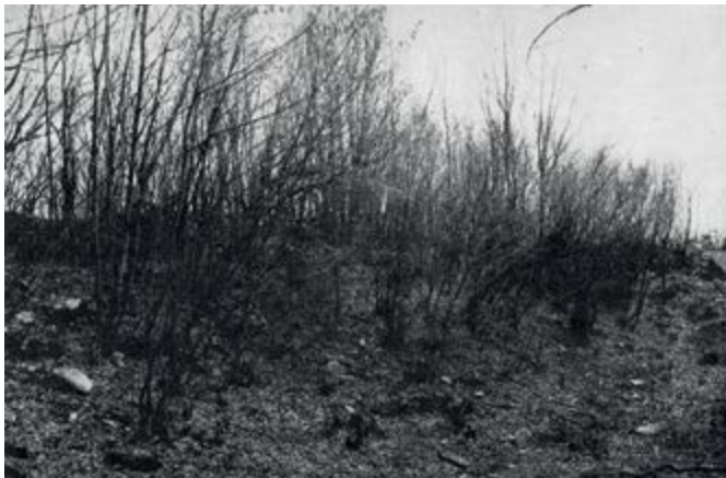
Figure 4. Medvedgrad castle before the conservation works in 1979
